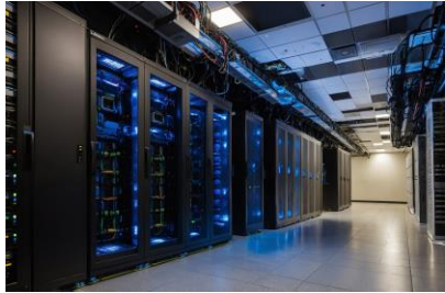
DESIGN & IMPLEMENTATION OF BACKBONE BMS ACROSS MULTIPLE DRC & DC LOCATIONS
